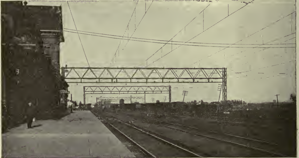
Overhead work in the yards in connection with the electrification of the St. Clair Tunnel.
