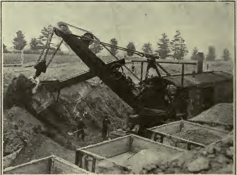
How the Railways try to keep up with the Western Grain-grower.—Steam shovel excavating 3,500 cubic yards per day on the Canadian Northern Railway.
