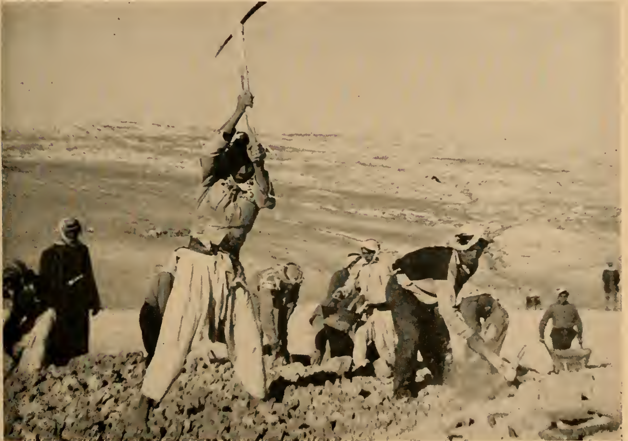
Jordanians at work on construction of an east-west highway system. Under the development assistance program, the United States is helping Jordan build more adequate road facilities to further the country's development as well as to give employment to thousands of Jordanians, including Arab refugees.
