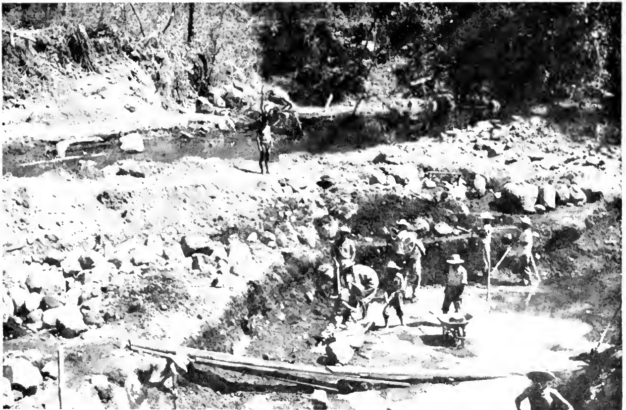
Foundations being prepared for a Pacific Slope Highway bridge across the Rio Bravo in Guatemala. The United States has earmarked $3.7 million to help complete this highway which will open coastal agricultural regions for development and help improve economic conditions in the country.
